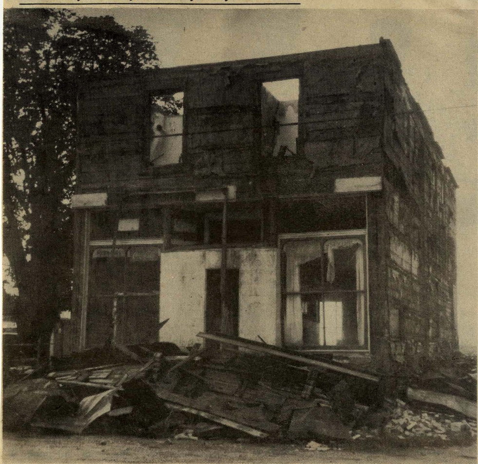
CLACHAN GENERAL STORE IS BEING demolished by owner Lloyd Brennan, the white brick veneer being removed recently, leaving the wooden frame to come down.
